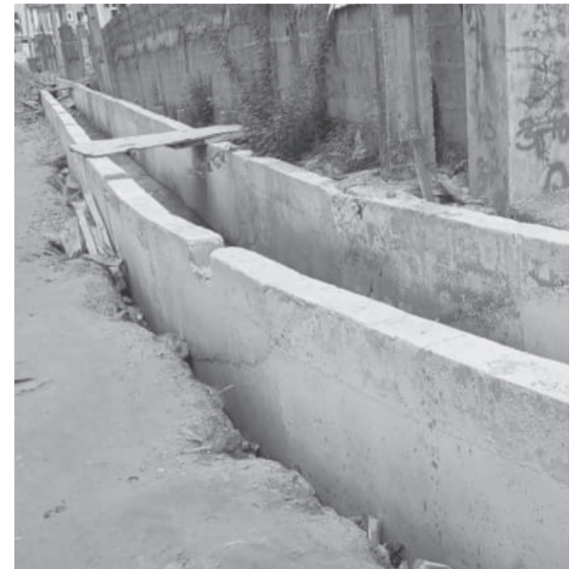
Greenfield community drainage
